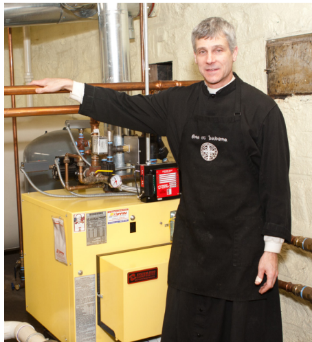
Br. Benedict proudly stands in front of our new boiler system
