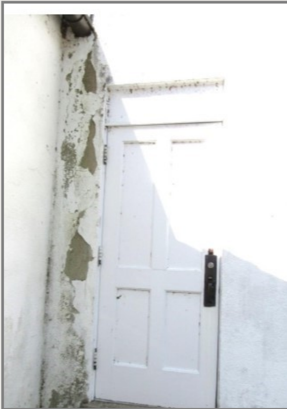
Example of extensive stucco damage
