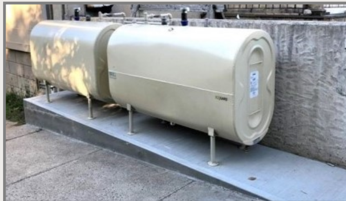
New oil tanks and pad
