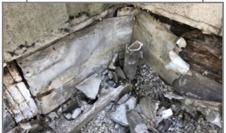
Damage to East side
