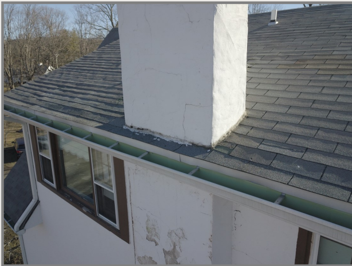
Roof, chimney and façade repairs needed on St. Joseph's
