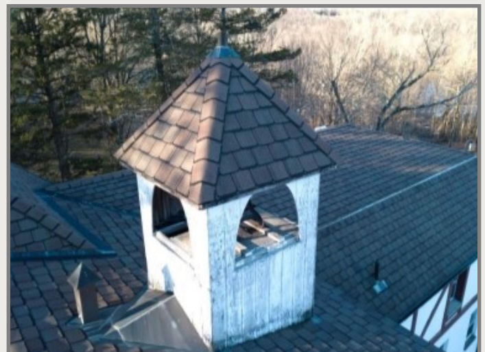
Retreat House bell tower in need of repair
