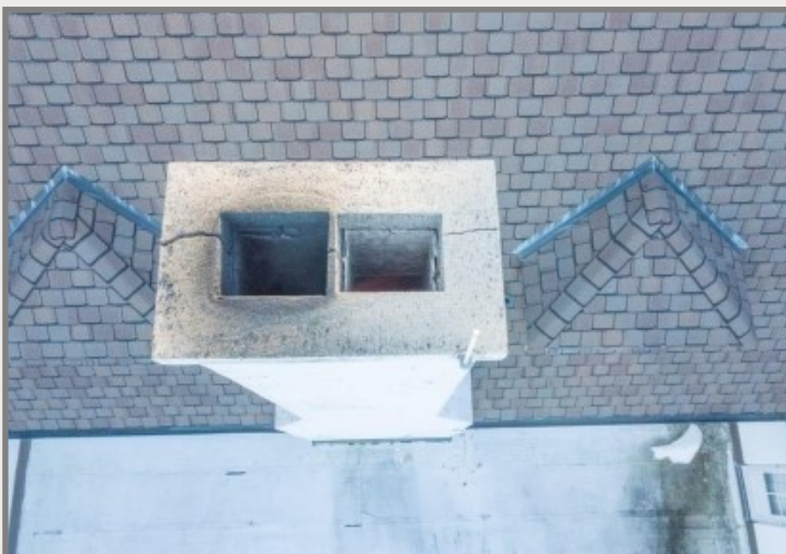
The many chimneys must be capped and tuck pointed
