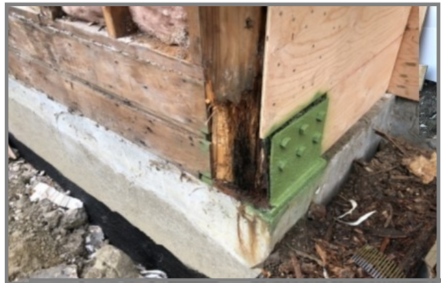
Damage to transept area
