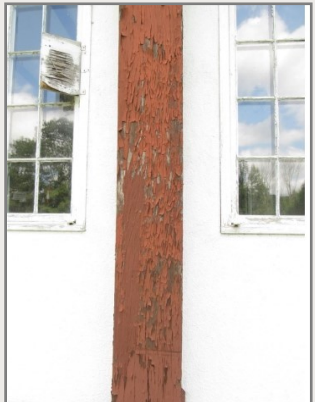
Damage to wood trim throughout exterior
